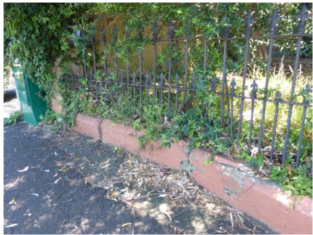
Picture 4 – Apparent subsidence affecting the front (south) boundary fence of 194 Oxford Street which is located at the corner of Oxford Street and York Road
